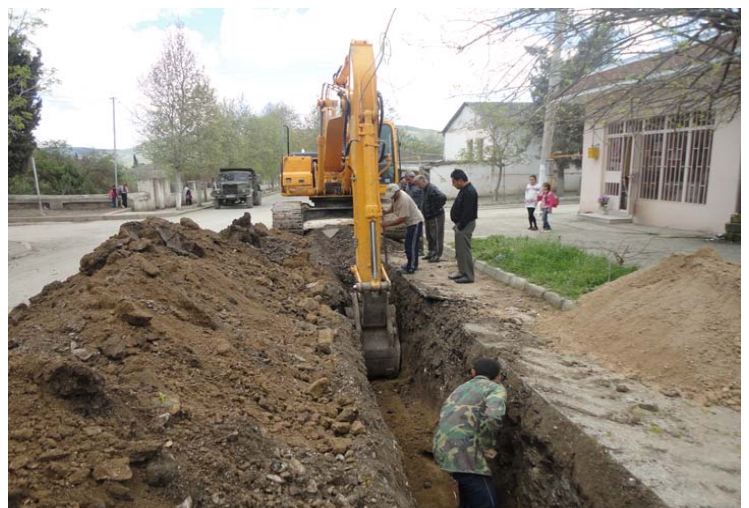
The sides of streets in the town of Martuni have been dug up to lay the new water network
