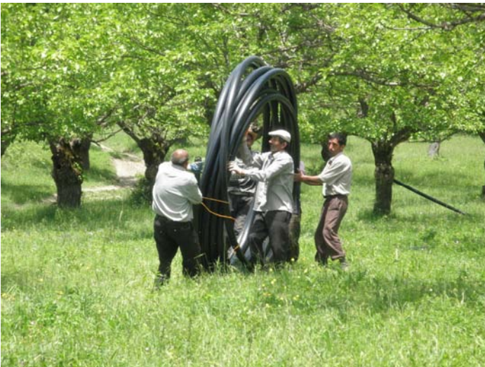
New technology allows workers to lay the water distribution network in Karmir Shuka quicker and with fewer issues.
